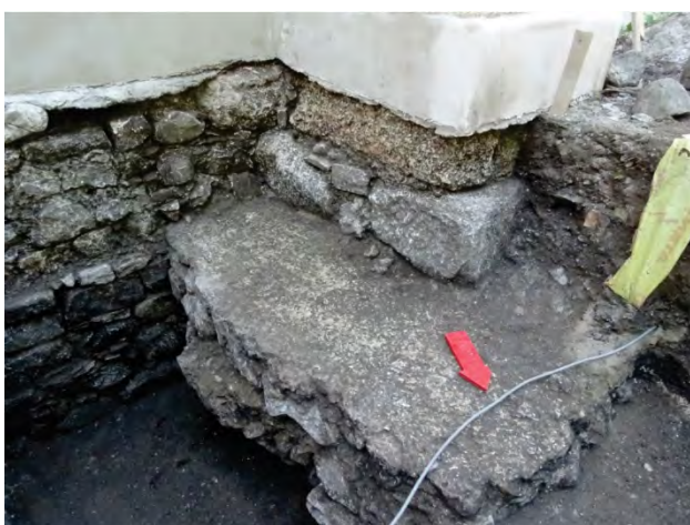
Figura 27. Fundația celui mai de vest contrafort perpendicular nordic / The foundation of the westernmost northern perpendicular buttress.
